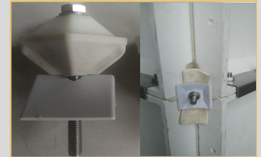
Leaking stoppage Plastic with SS304 bolts & rubber
